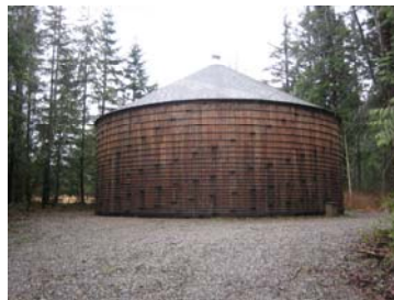
C G Engineering Greg Guillen, PE SE Camp Waskowitz Water Tank Repair, Highline School District
