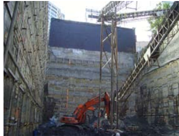
Golder Associates Richard Luark, PE Escala Condominiums: 94 Ft Deep Excavation, Lexas Companies, LLC
